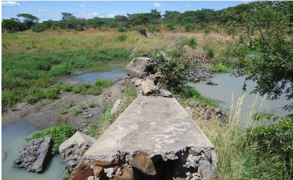
Figure 3.7: Damaged Dam on the Rungwa River.
